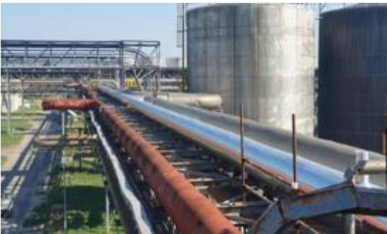
Views of the new P3 steam pipeline route on bridge C of DN 400
